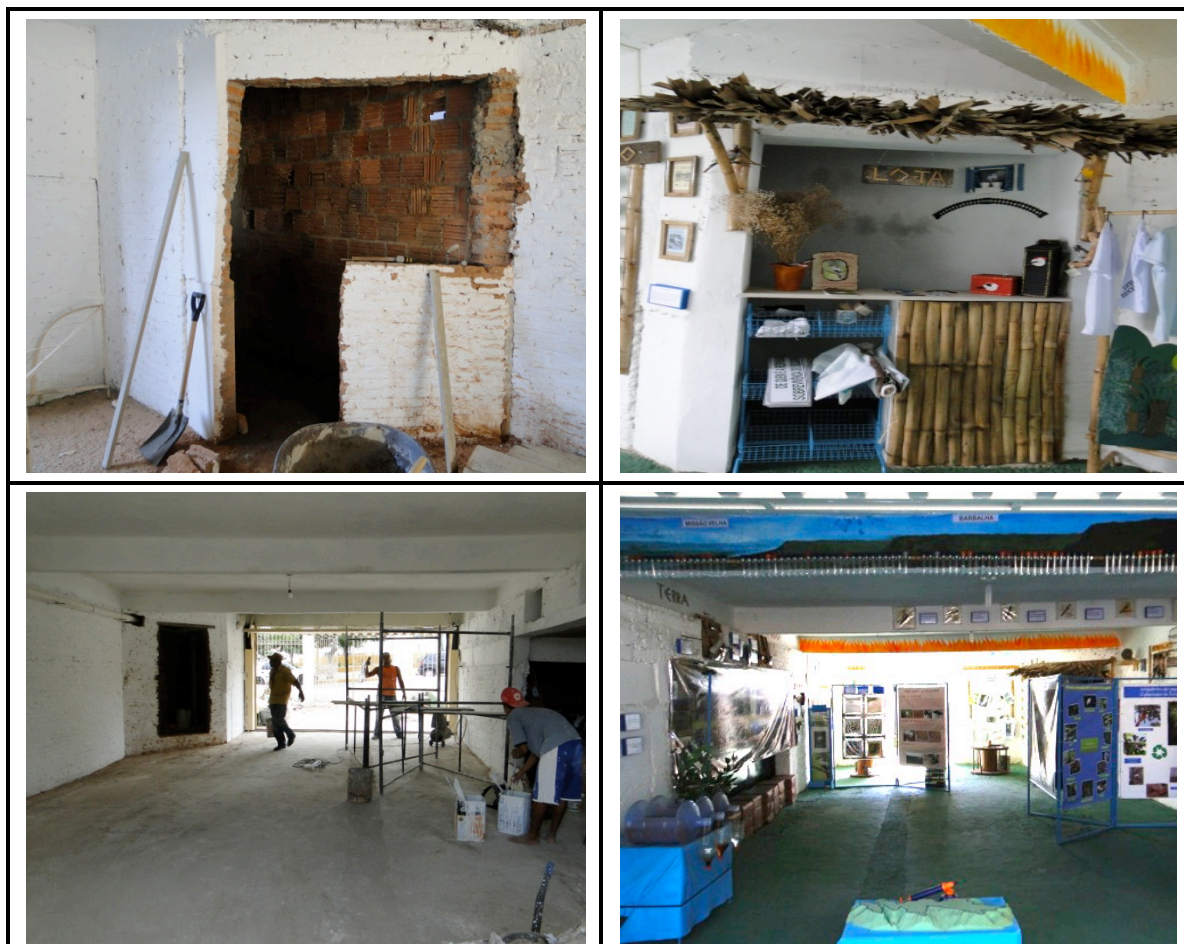
Figure 28. Various stages of construction and recuperation of the ICC garage area to transform it into parts of the Araripe Manakin Education Space ( Espaço Soldadinho-do-araripe - ESA). Top: the ESA store space before and after; Bottom: the main parlor and exhibition space before and after.
